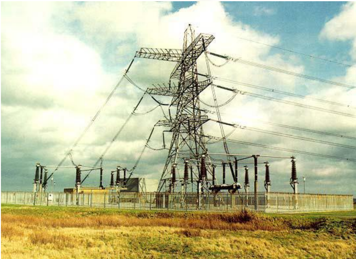
Figure 3: 400kV Transition compound
