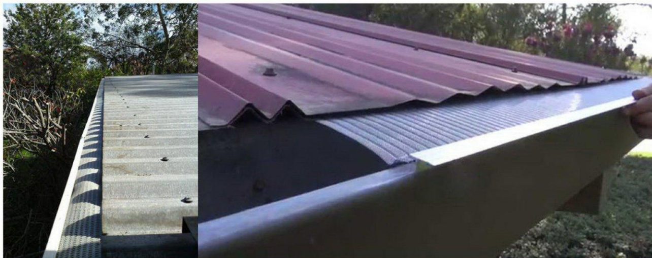
Figure 8: Gutters need to be cleaned out regularly; installation of gutter guards will reduce maintenance requirements
