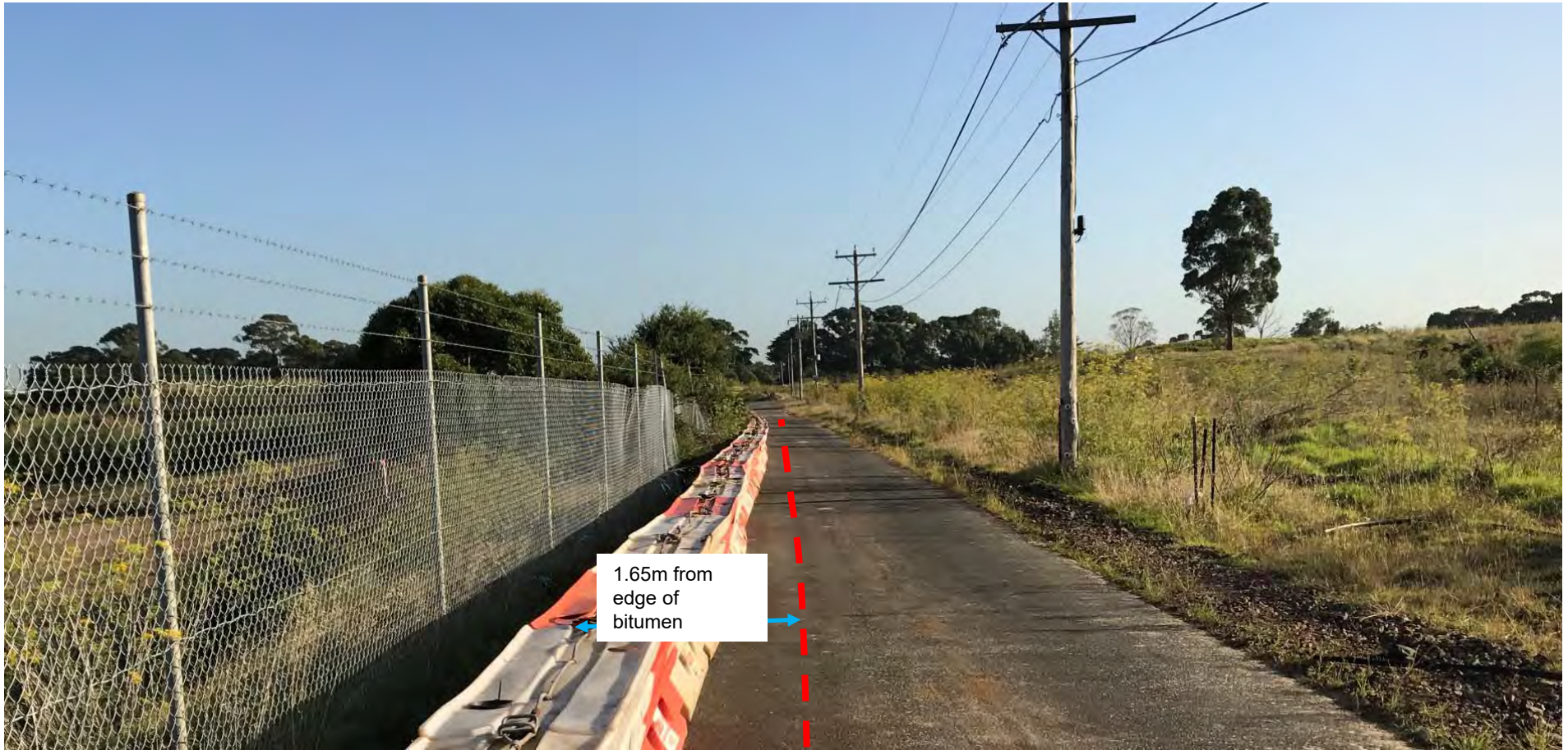
Exclusion Zone with 1.65m offset measured from the edge of the bitumen to be applied over a 57m length as shown in D03_Rev03. The barriers are to be located so that the truck wheel tracks are to be at least 1.65m from the edge of the bitumen.
