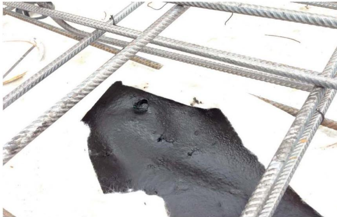
Photograph 2 – Punctured membrane. Based on size of puncture, cause possibly due to steel. Puncture and sealed with Liquid Boot roll grade.
