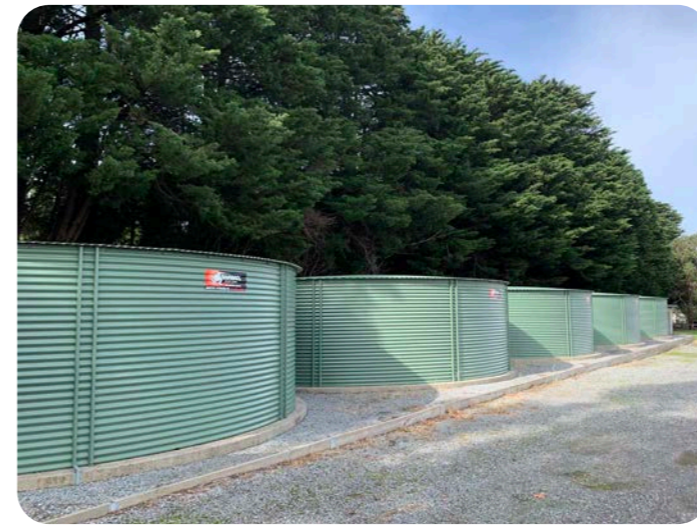
Water tanks on eastern boundary
